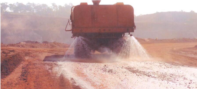
Dust suppression system by water sprinklers procured from BEML having capacity of 28000 litres.
