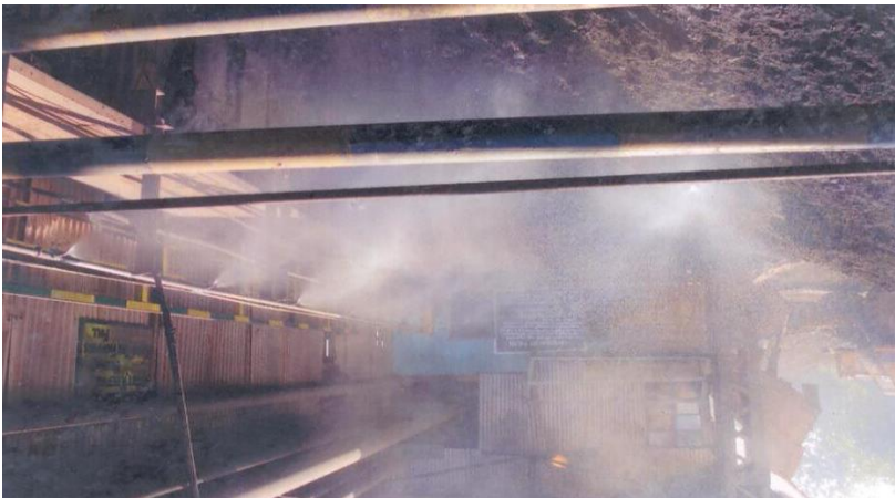
Water spray nozzles have been fitted at all transfer chutes and hopper to control dust pollution
